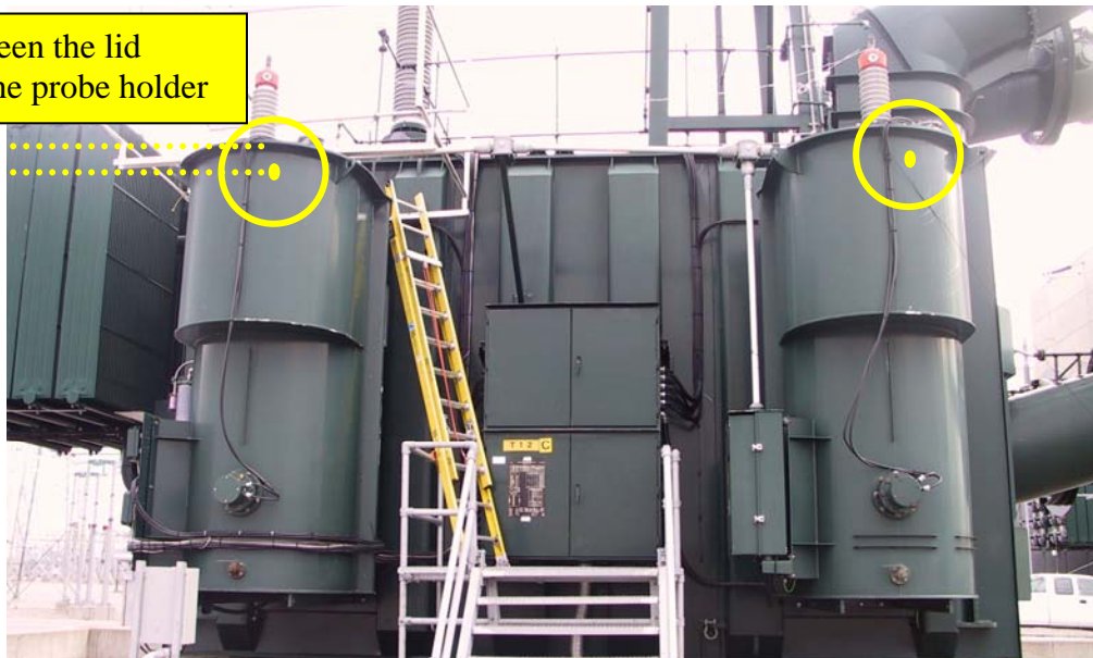
Figure I.3: ABB UCD with cylinders multiple in separated tanks
