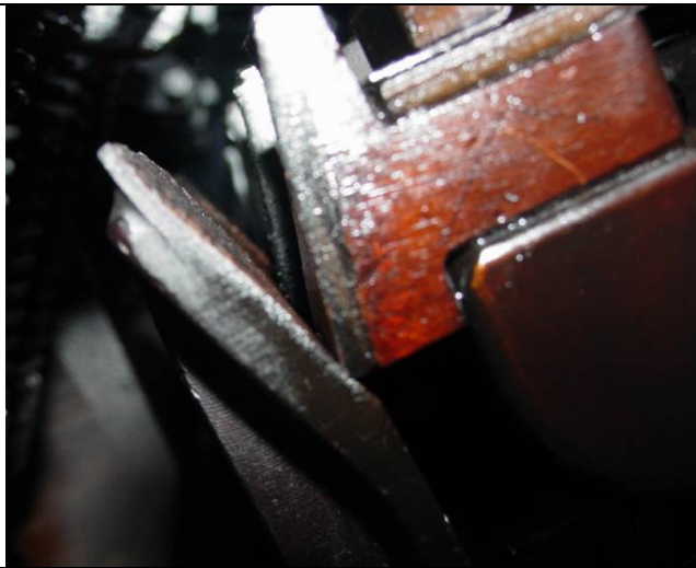
Worn contacts (before repairs)
