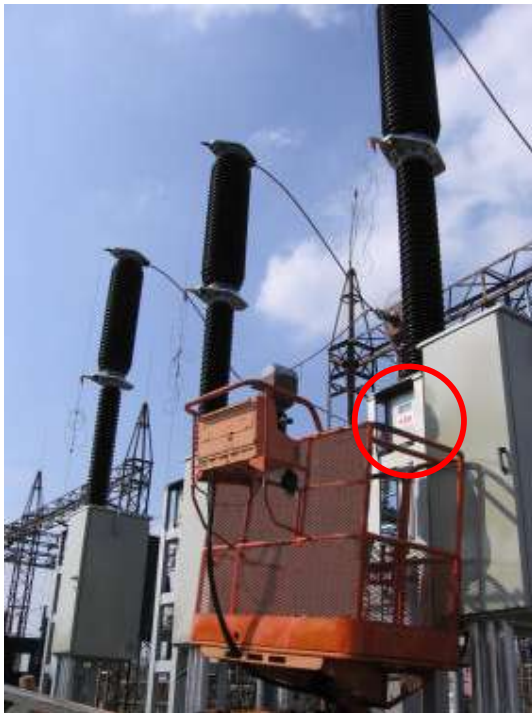
General view of the breaker
