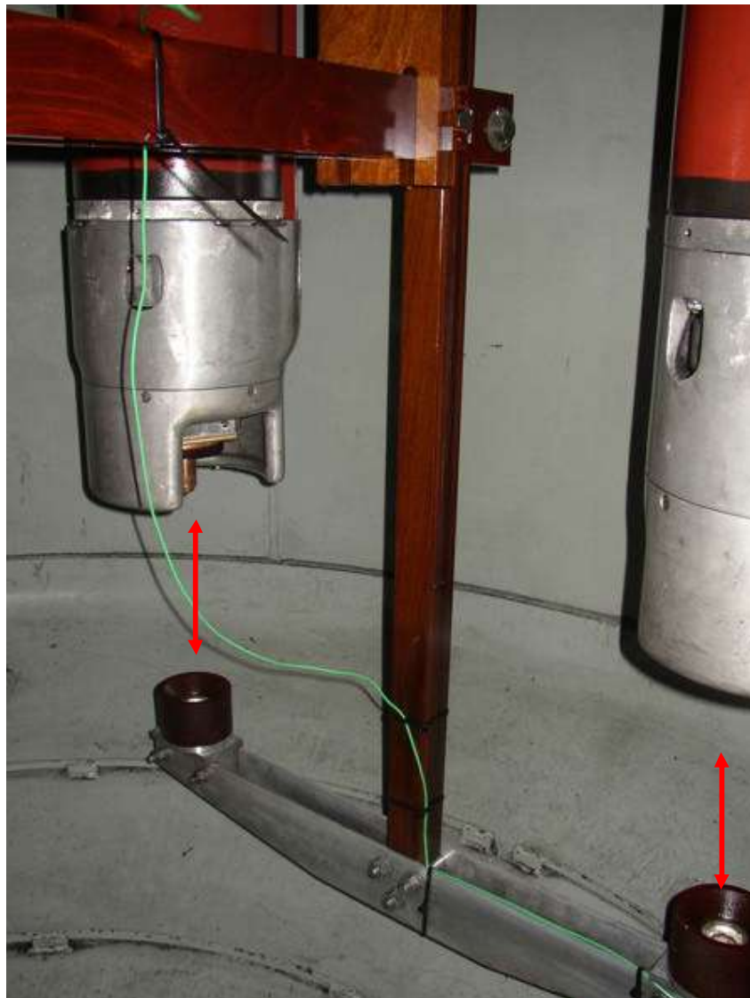
Bulk oil breaker
