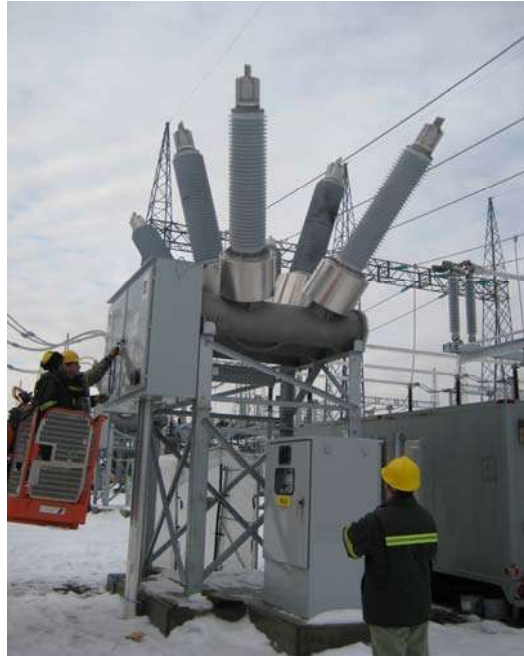
(Fig 1) Circuit breaker
