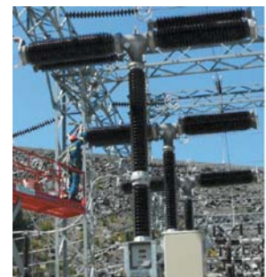
Fig 10 HPL SF6 circuit breaker
